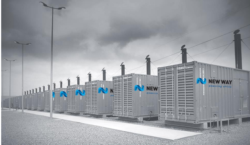
Large Generator Prime Power Plant (Sales and Rentals)
